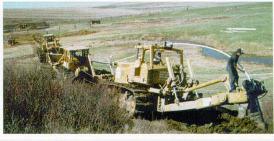
Figure 15: Two Fiat Avis F040's and a Caterpillar D-8 combine their 1210 HP to plow-in a rural water pipeline across a bone-dry pasture near Milk River, Alberta (PFRA photo 615302-2). The water source for this 90+ farm distribution system is a single well shown pump tested at 250igpm. (PFRA photo 61415-2).
