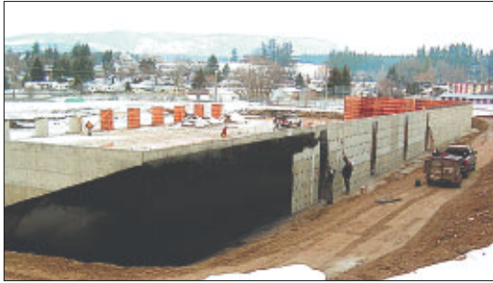
Construction is proceeding on the new Armstrong/Spallumcheen Recreational Complex, which will include an NHL-sized arena and is expected to play host to local and international athletes once completed.
