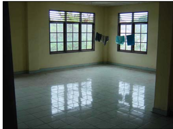
Figure A6.2: One of the many empty office rooms in the water supply enterprise transfer station building funded by ADB.
