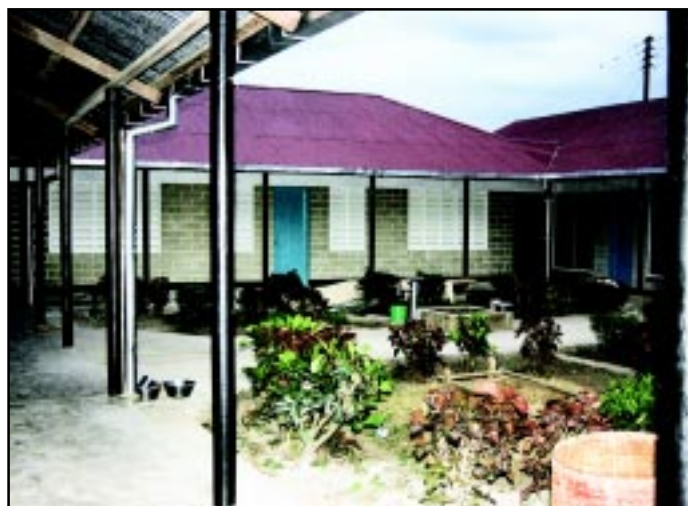
The new looks of a rehabilitated health centre at Ngerengere, Morogoro Rural District.
