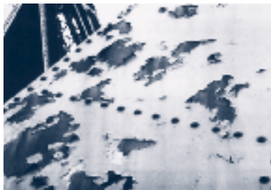
There is a problem with corrosion on the unrepaired part of the bridge and the paint is in poor condition.
