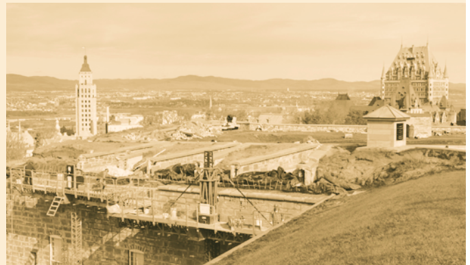
The Citadel in Quebec City is undergoing a $20 million wall restoration. This work is done with the full cooperation and assistance of Parks Canada and the Federal Heritage Buildings Review Office (FHBR).
