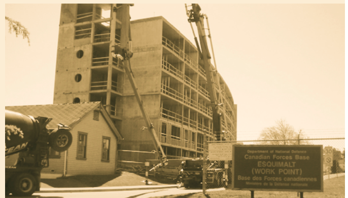
Construction of the new Naval Officer Training Center (NOTC) at CFB Esquimalt, British Columbia is currently underway with completion scheduled for the fall 2004. DCC is providing contract management and quality assurance services.
