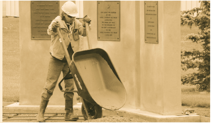
As part of the general maintenance work done at Bushell Park, Saskatchewan, DCC manages work orders with standing offer contractors. Above, a contractor is building a monument dedicated to the fallen airforce heroes of 15 Wing Moose Jaw.
