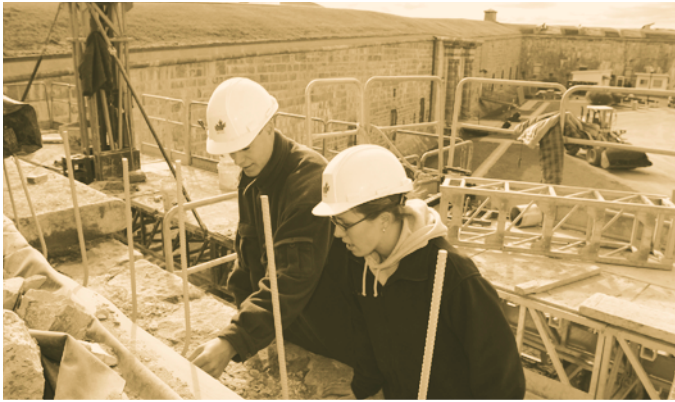
Two of DCC's technical staff inspect the masonry at the Citadel in Quebec City.
