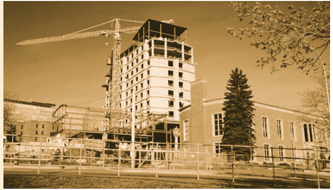
Construction of the Chiefs and Petty Officers and Officers Facility commenced last year at CFB Halifax in Stadacona. DCC is providing procurement and contract management services.
