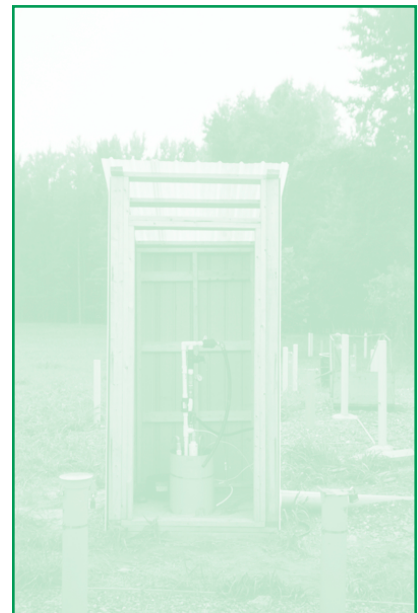
A recirculation and chemical-injection well at the site of the pilot-scale groundwater remediation study at the Aberdeen Proving Grounds.
