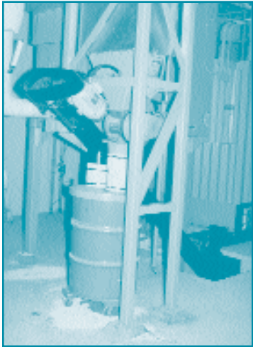
Ash Removal Conveyor and Storage Drum: Automated BCS
