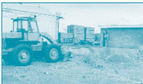
Mobile Loader Delivering Fuel to In-ground Bin
