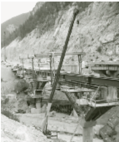
Construction of 5-Mile Yoho Bridge in Kicking Horse Canyon, British Columbia—Strategic Highway Infrastructure Program Project Photo: Transport Canada
