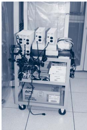
Battery backup power source
