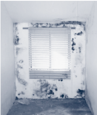
Mould contamination inside a home on-reserve
