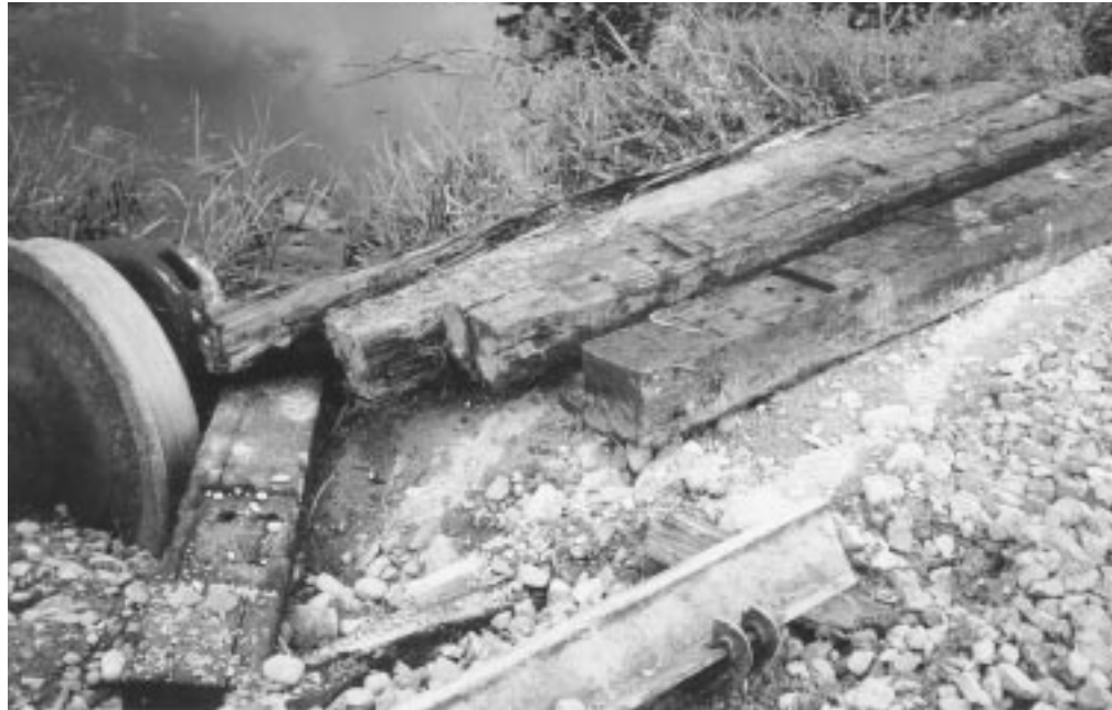
Broken ties, a broken rail, and part of a wheel set lie on the shoulder of the track.
