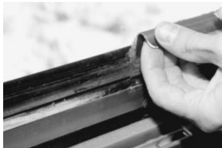
The size of the little metal handle on the emergency exit windows limits the force that can be applied to it. The handle also causes the windows to jam on the window frame.
