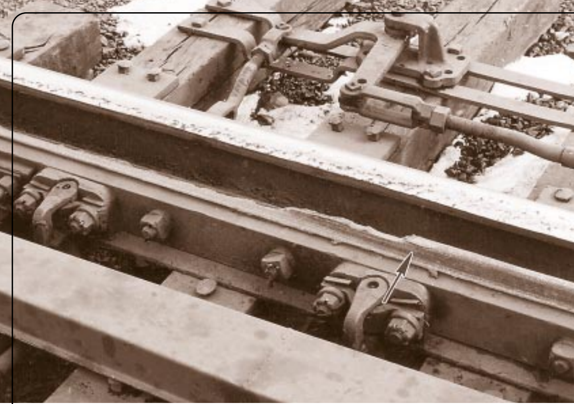
View of the missing section of the running surface of the switch point. The arrow points to a crack in the rail adjacent to missing head fragments.
