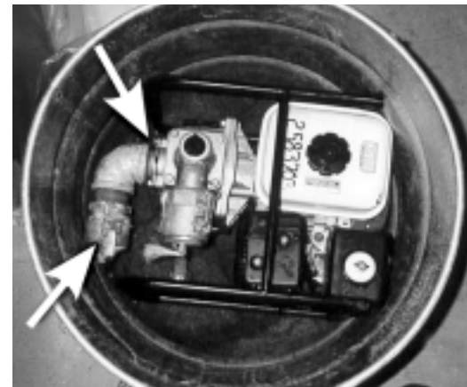
CCG helicopter-delivered Honda unit, tightly fitted into the drum. 'A' indicates contact point of pump with drum. Location of suction flange fracture is shown at 'B'.
