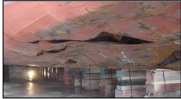
Figure 8. No. 1 starboard double bottom ballast damage
