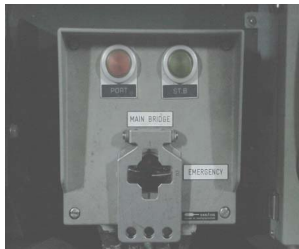
Figure 3. Emergency Remote Control Transfer Switch
