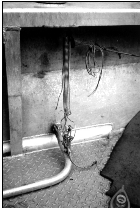
Photograph 4. Disconnected remote stop device (hold-to-run control).
