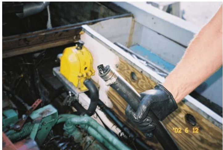
Photo 3. Electrician's tape protruding from failed joint in engine cooling hose
