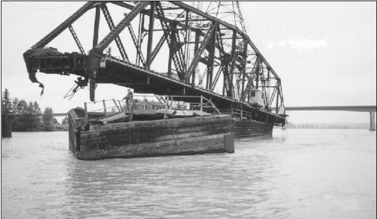
Figure 4. Damaged nose of protection pier deflected to north.
