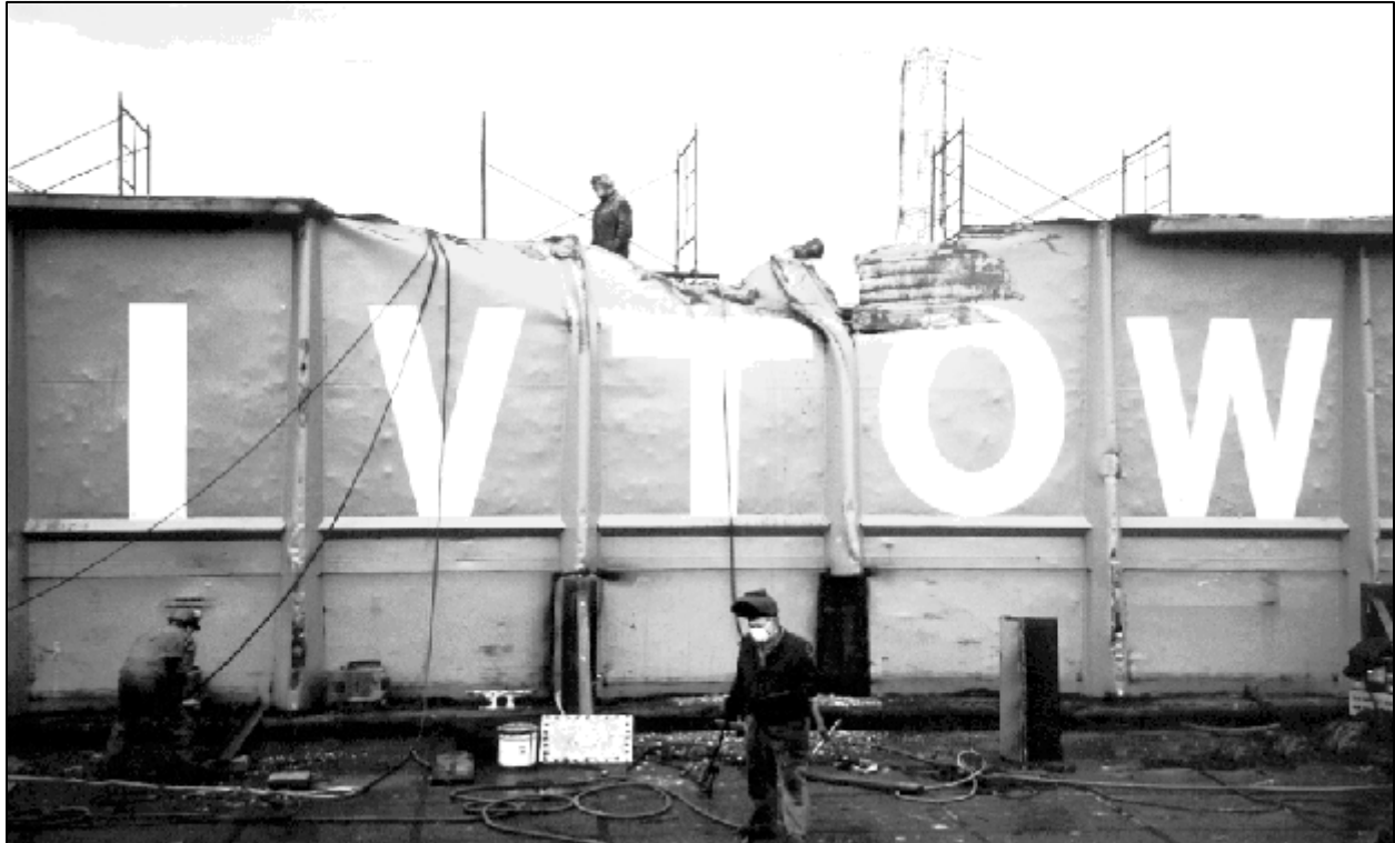
Figure 3. The chip barge Rivtow 901 with damaged starboard box-wall under repairs.
