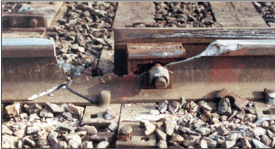
Figure 5 - The broken rail at the point of divergence.
