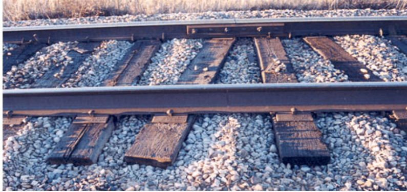
Photo 2. Skewed ties at joint
