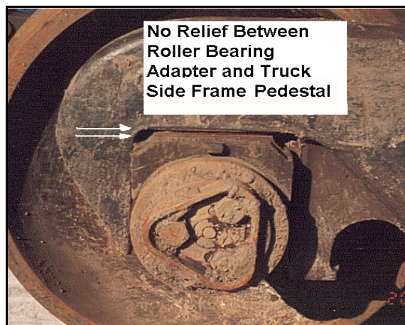
Photo 3. Lack of adapter relief on CGTX 64098; also note marks on wheel plate due to contact with non-ferrous materials (e.g. ballast and ties).
