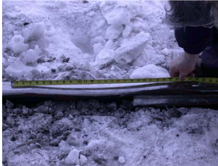
Photo 1. Crushed rail head
