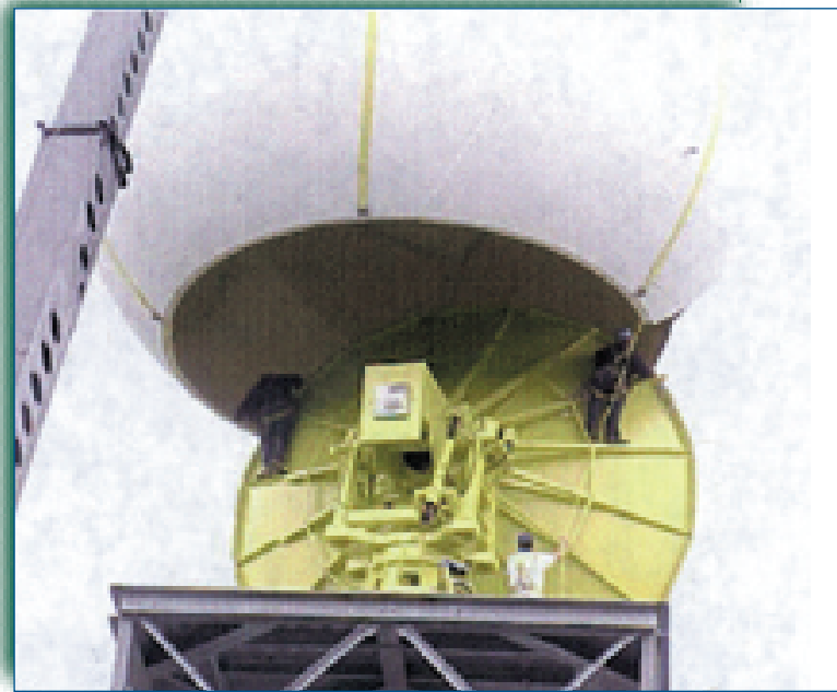
▲ Weather radar installation in Franktown, Ontario
