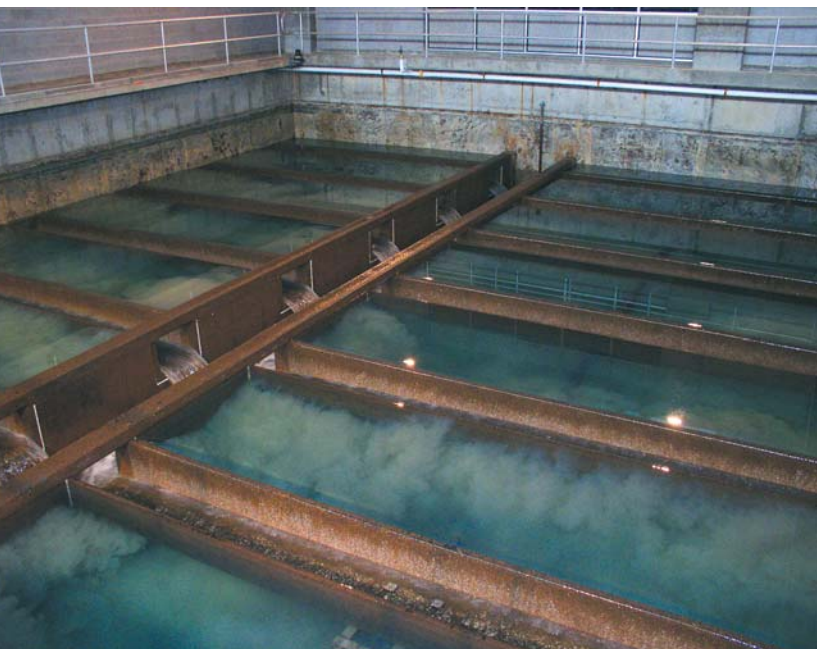
Backwashing sand filters in a water treatment plant.
