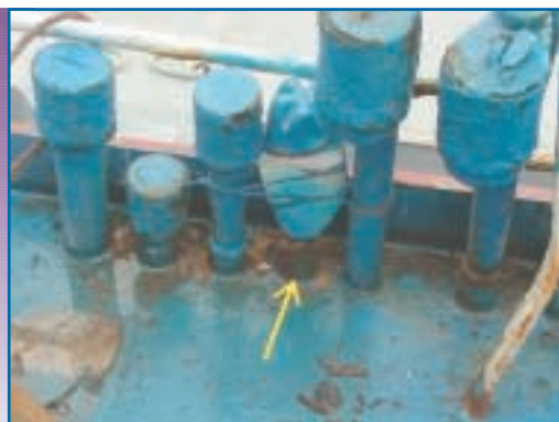
Head of a ventilation pipe replaced by 2 litre plastic bottle
