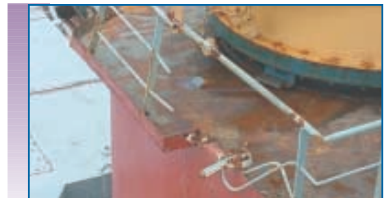
Guardrails corroded and broken off on ship's crane platform
