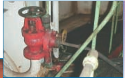
Fire hydrant unable to be used with fire hose
