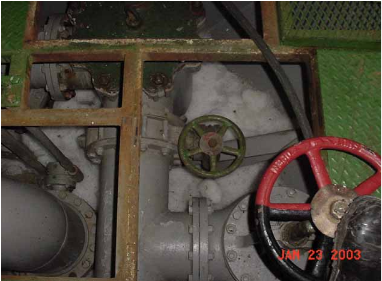
Figures 3.7A – Frazil ice accumulation at the bottom of engine-room bilges after numerous seawater strainer cleaning
