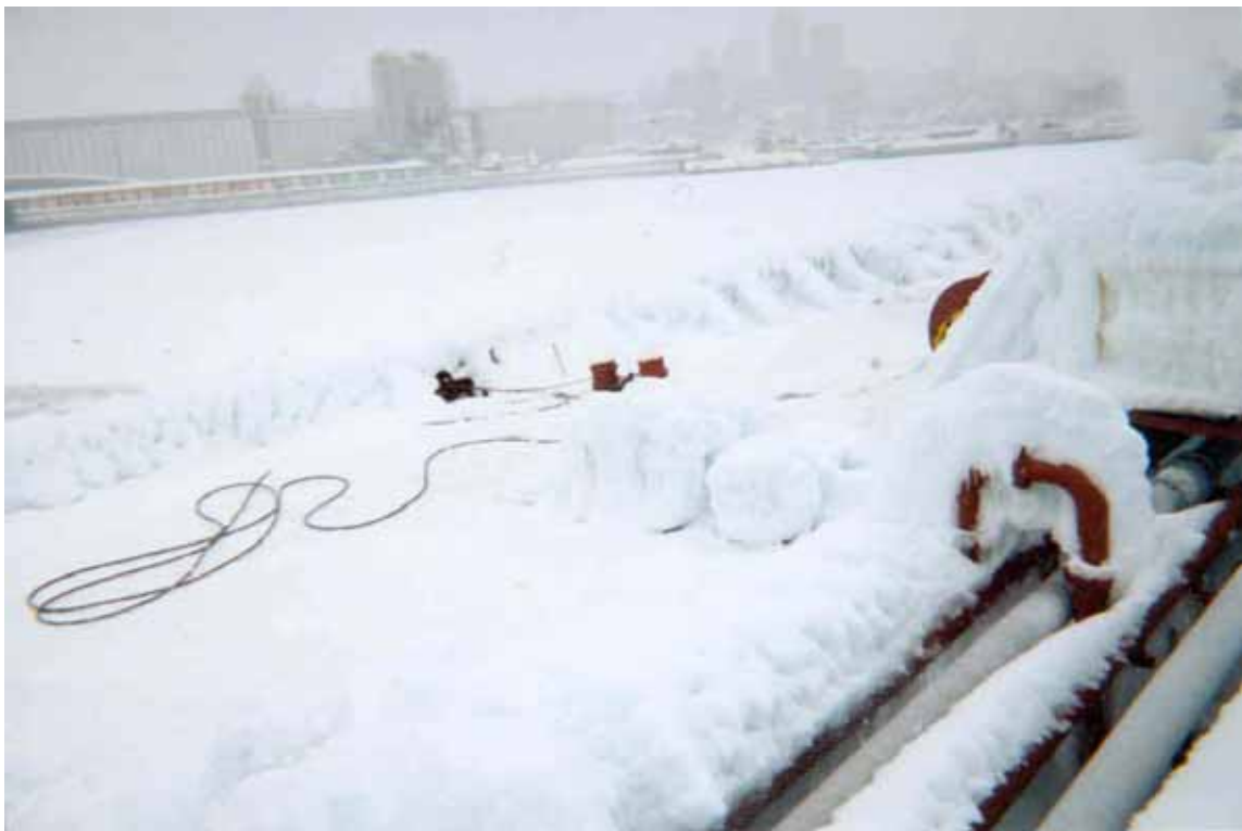
Figures 5.3F– Deck, piping and valves inaccessible
