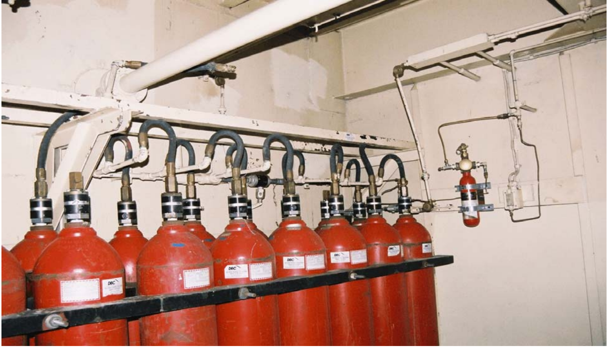
Photo 2. Bank of CO 2 cylinders and distribution manifold
