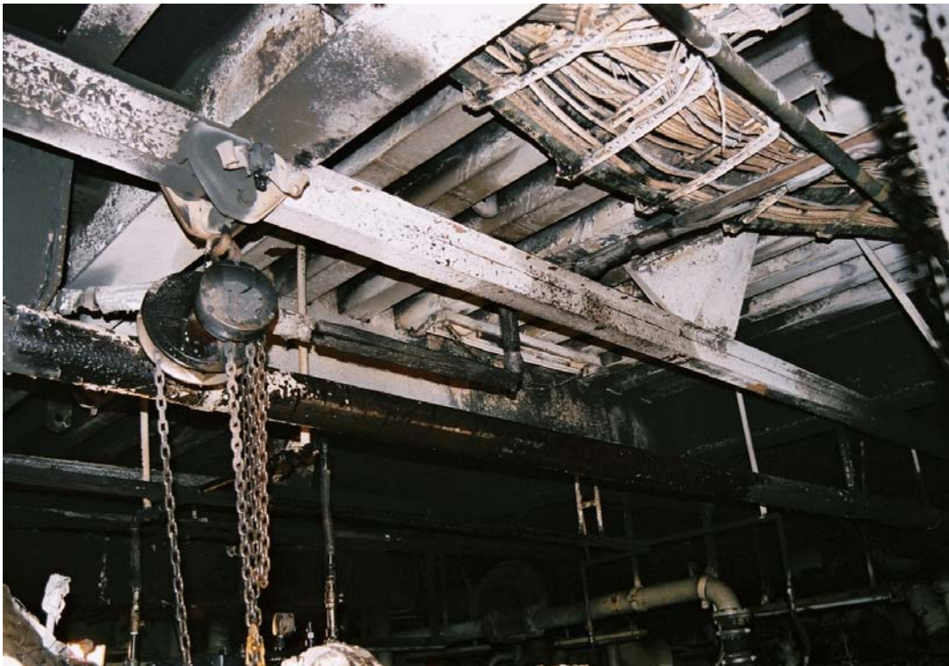
Photo 3. Damage to engine room and electrical cables
