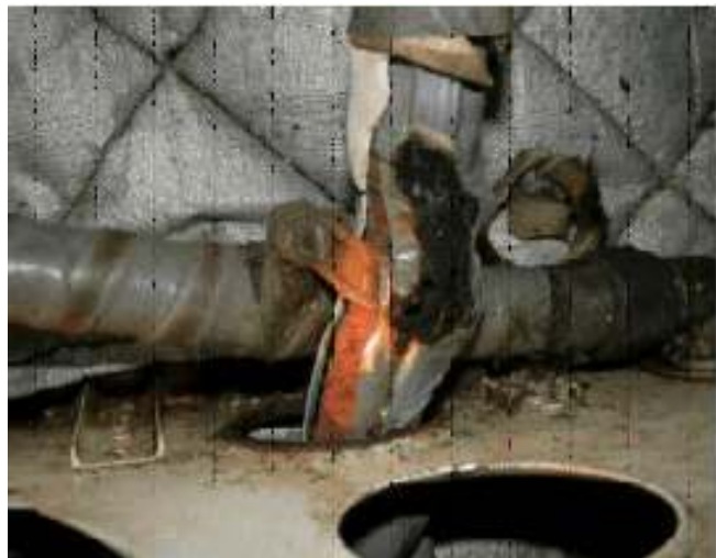
Photo 5. Burned heater ribbon behind aft wall
