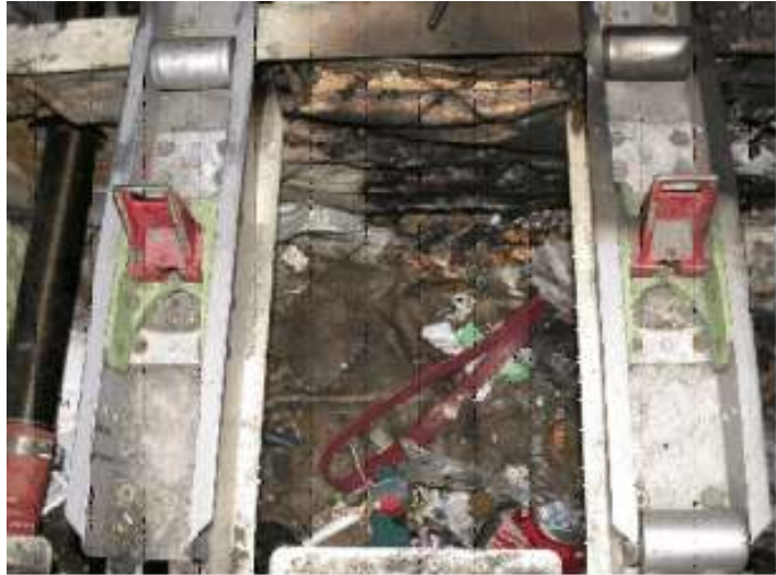
Photo 4. Contaminated insulation blankets and debris
