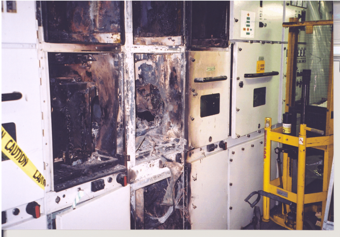
Photo 1. View of DG 2 circuit breaker and relay consoles. DG 1 and bus-tie breaker consoles are on either side.
