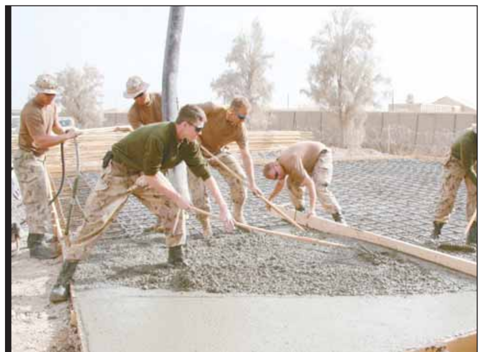
Troops from 191 AEF (Comox), 192 AEF (Abbotsford), and PNCT (Esquimalt) pour concrete for an extension to the TOC building in Kandahar, Afghanistan.
