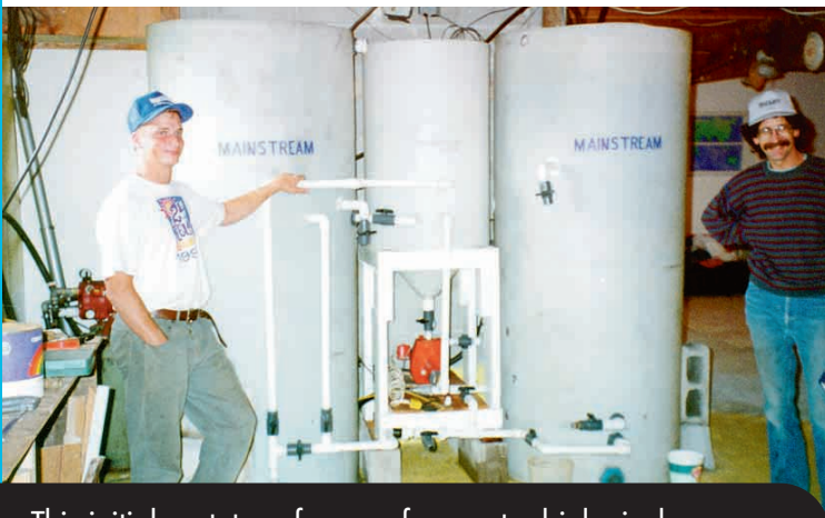
This initial prototype for a surface water biological treatment system was installed for a farmer in December, 1993
