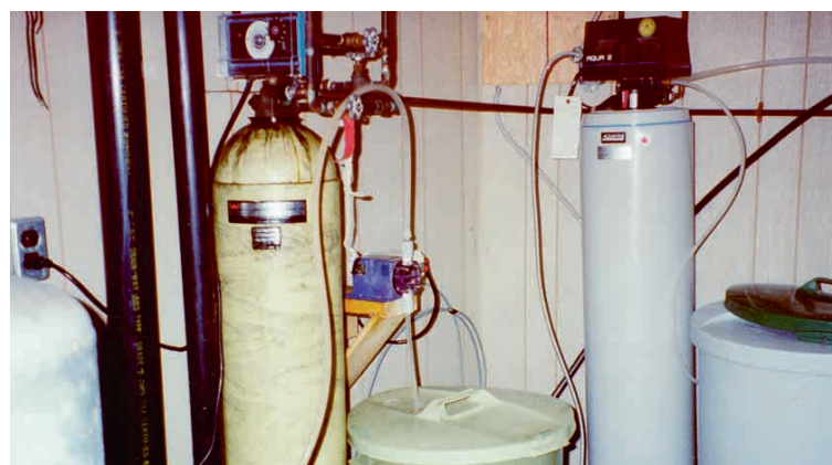
A common primary water treatment system for Prairie farms is a chlorinator, carbon filter and softener
