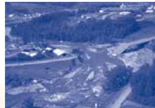
Collapsed bridge and eroded banks along the Rivière à Mars, Saguenay Valley, Quebec, following the catastrophic flooding of July 1996. Date of photograph: July 27, 1996.
