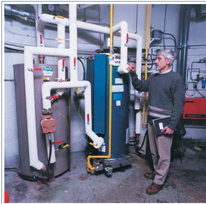
Advanced Integrated Mechanical Systems
