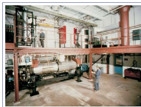
1 MW t Thermal Rotary Kiln
