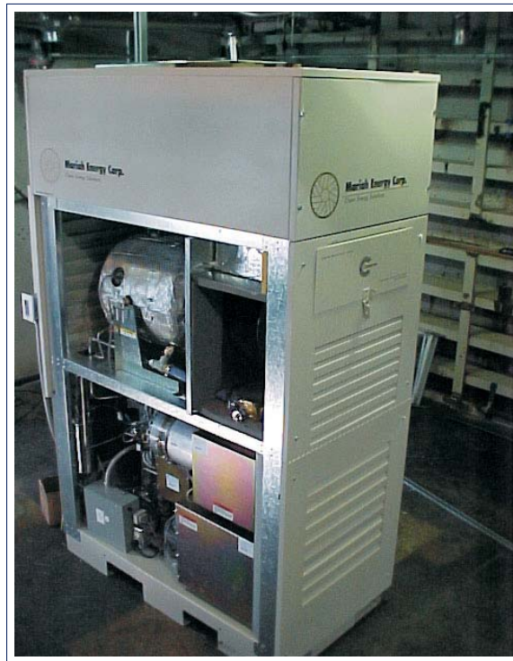
Mariah CHP Unit at CETC
