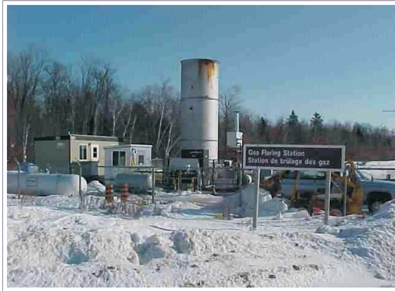
Honeywell Microturbine at Trail Road Landfill Site, Ottawa, Canada
