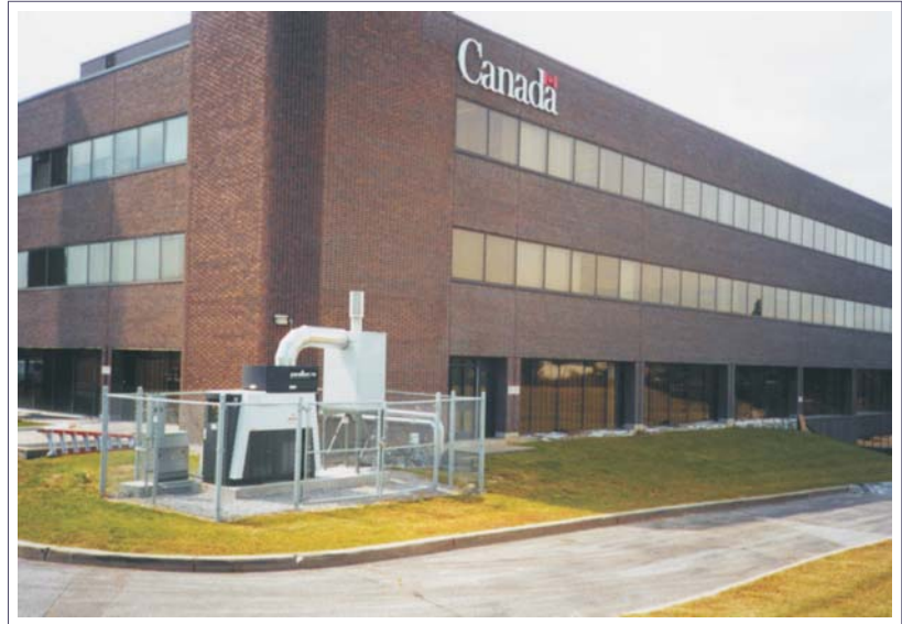
Honeywell Microturbine with an Unifin Heat Recovery Unit at Health Canada Building, Toronto, Canada
