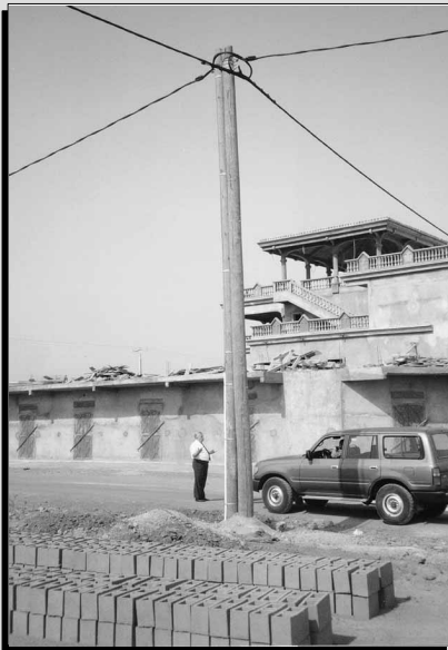
View of an electrical pole installed as part of a CIDA project to renovate and restore the electrical distribution system in Bamako, Mali.
