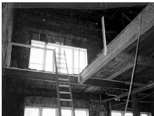
Canada Business Service Centre at 338 Charlotte Street, Sydney, CBSC undergoing initial building renovations (see paragraph 17.17).
