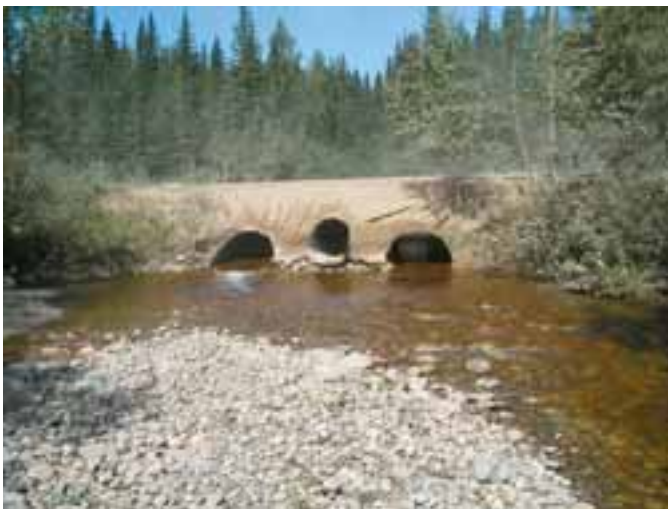
Fish Creek, near Hinton, AB: before reparation
