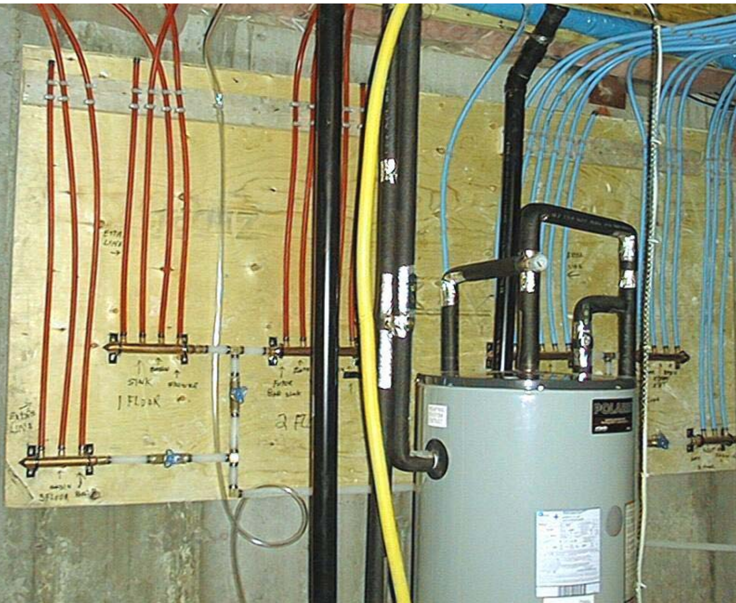
Polaris high efficiency direct vent water tank and plumbing manifolds in Flex Unit
