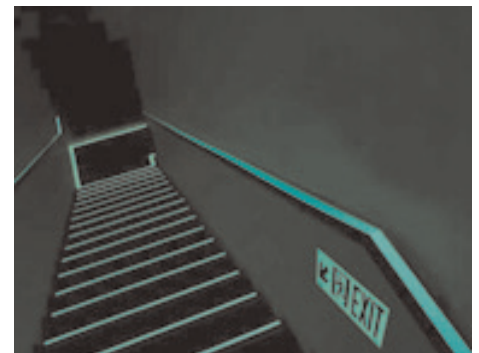
Photoluminescent exit path marking following Reference Standard 6-1 required by New York City Building Code 2004
