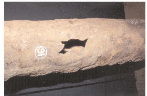
Failed cast iron distribution main
