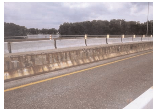
The Vachon Bridge parapet wall 20 years after construction. It shows significant corrosion prior to reconstruction and installation of a corrosion inhibiting system.
