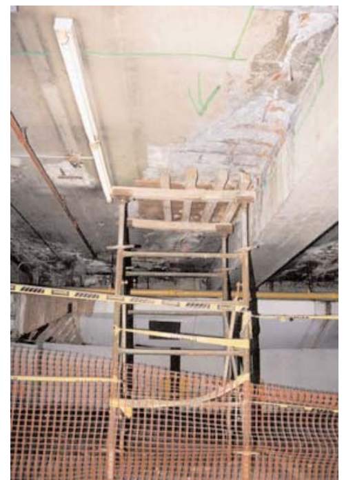
Typical Deterioration Found in Parking Garages
