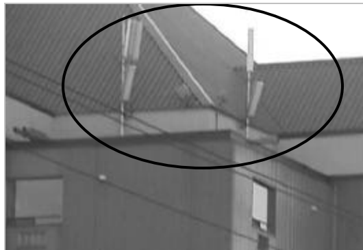
Figure 10. Cellular antennas mounted on a building
