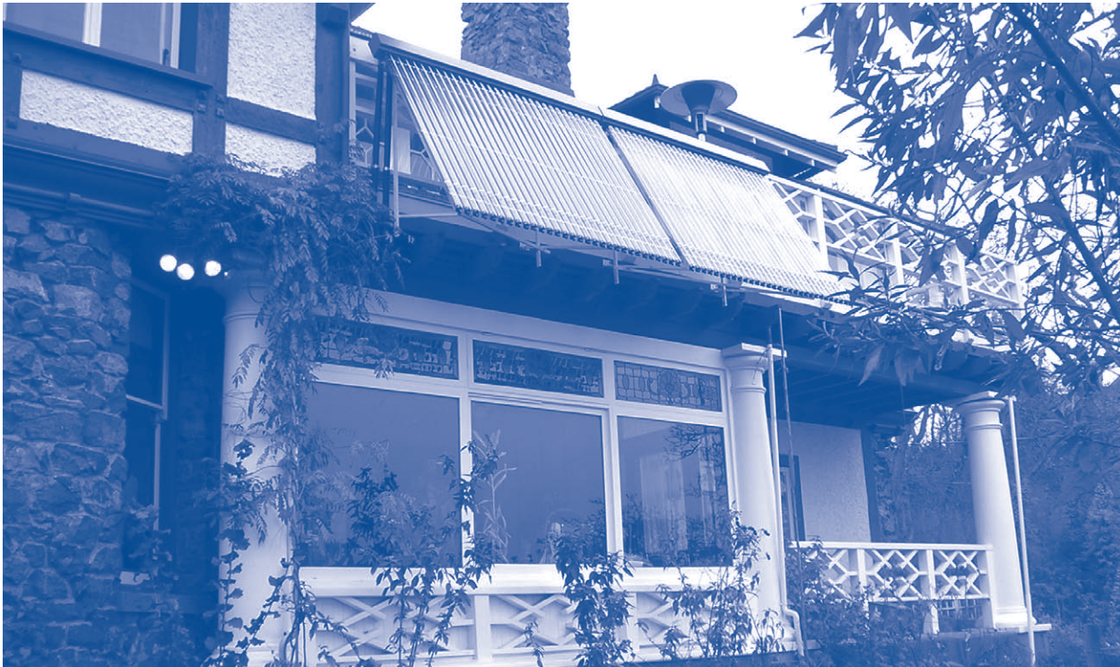
Solar panels are used to heat water in homes.
