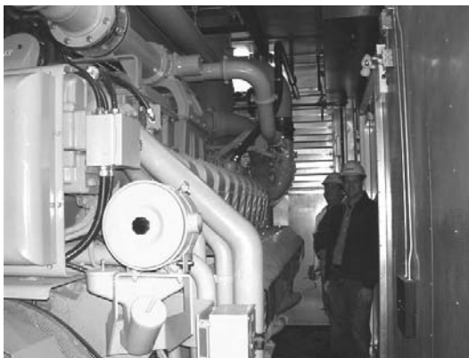
FIGURE 4.3.2 Cloverbar Landfill Gas Site, Edmonton, Alberta
