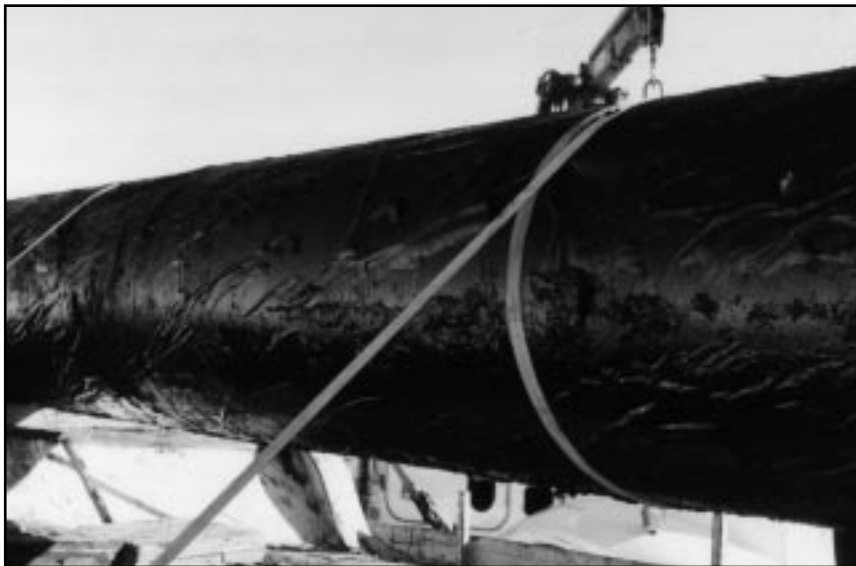
Figure 3.10 Polyethylene tape coating in poor condition due to wrinkling
