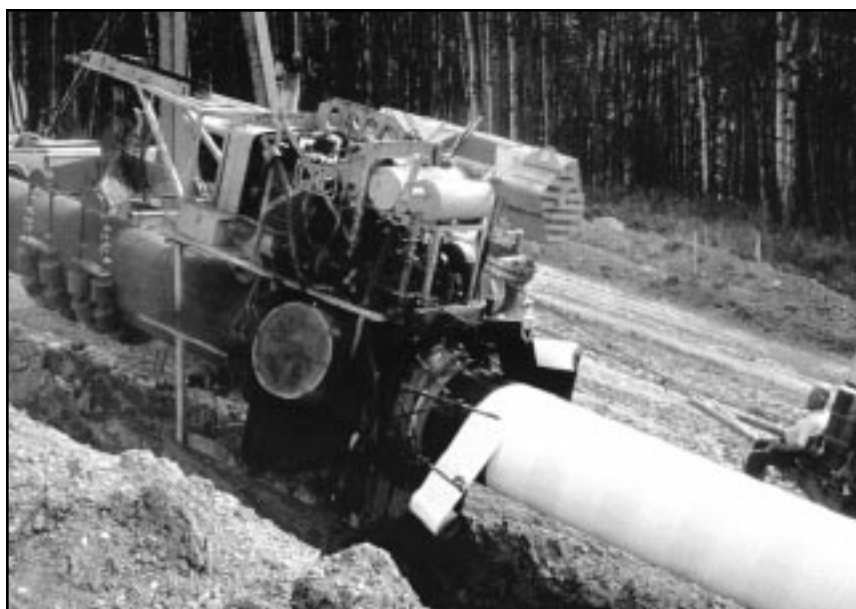
Figure 3.6 Tape wrapping machine
