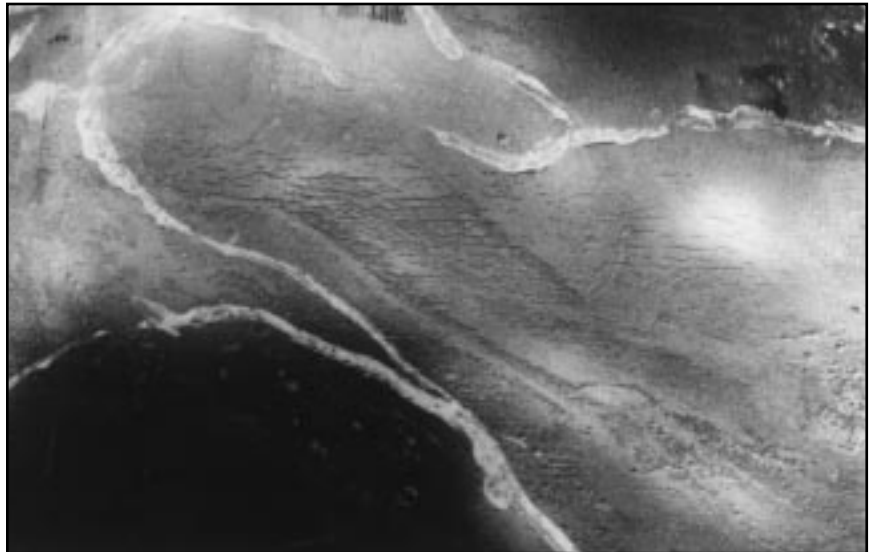
Figure 3.12 SCC cracks under spiral polyethylene tape overlap
