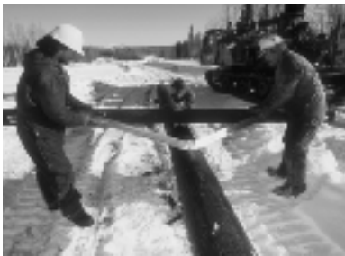
Workers mount a crossarm on a wood pole, which is used for the transmission line.
