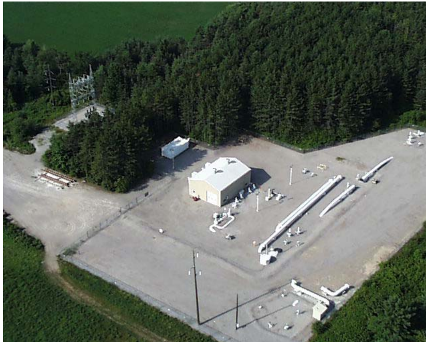
Photo 3-1 Pump Station – Example
